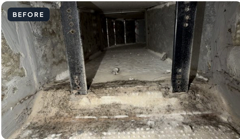
Living room supply duct
